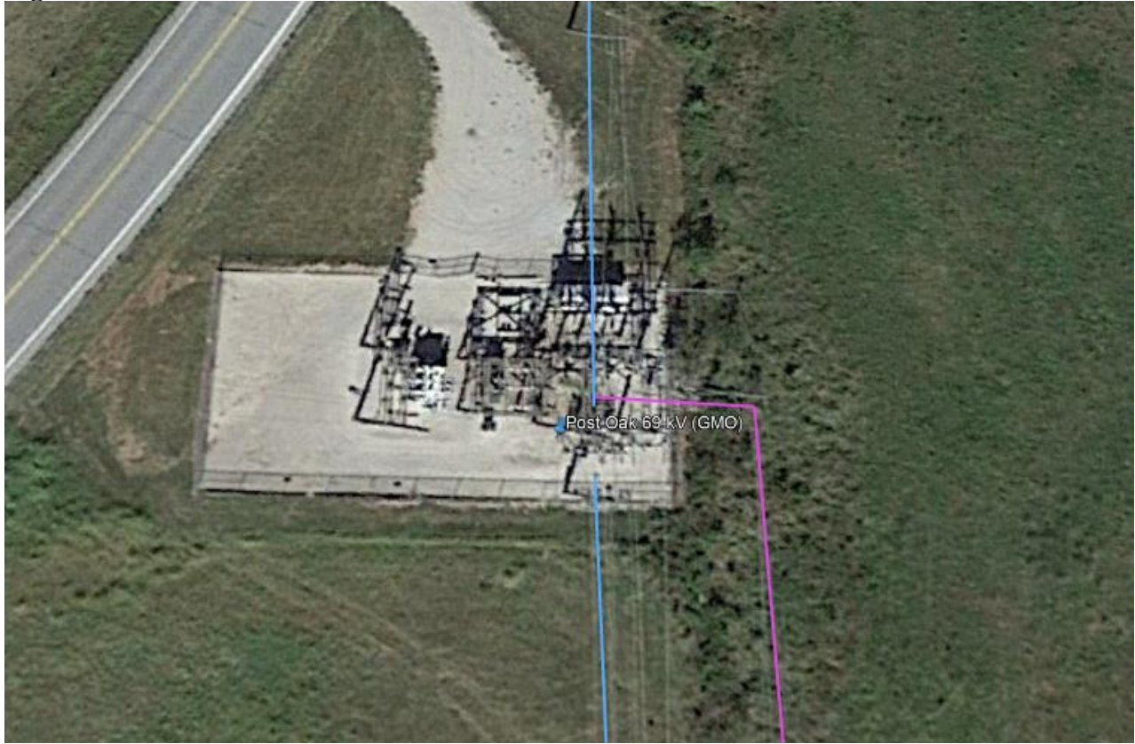
Figure 4 – Post Oak – 69kV Transformer
